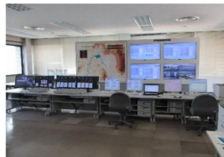
3Floor Operation Room
